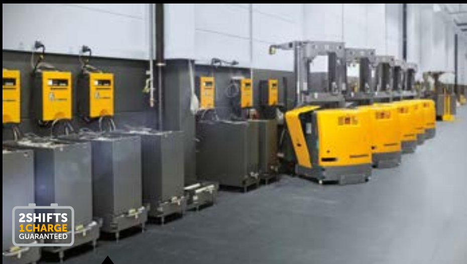
Charging lead-acid batteries in a separate battery area.
